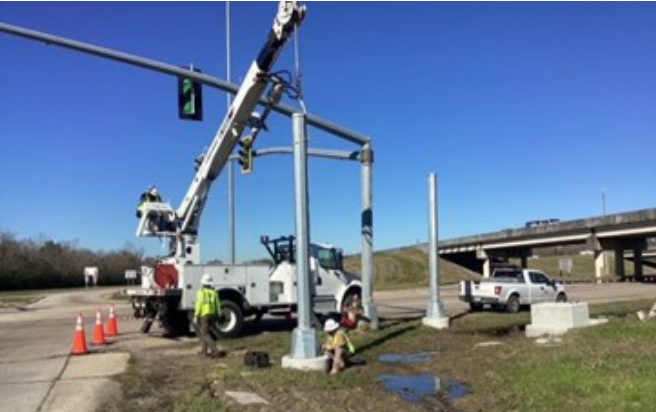
GEC is providing field inspection services for the installation of upgraded traffic signals featuring flashing yellow arrows in District 61.
